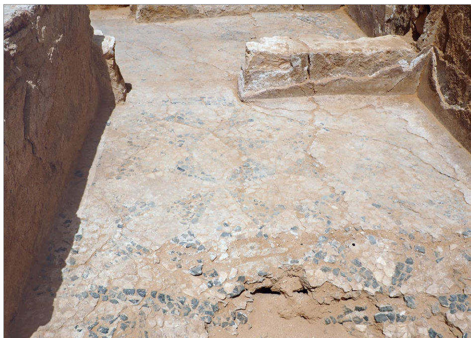
Fig. 1. Cracked walls and mosaic floor in the H.39 bathhouse, view from the east (PCMA UW | photo K. Jakubiak)
