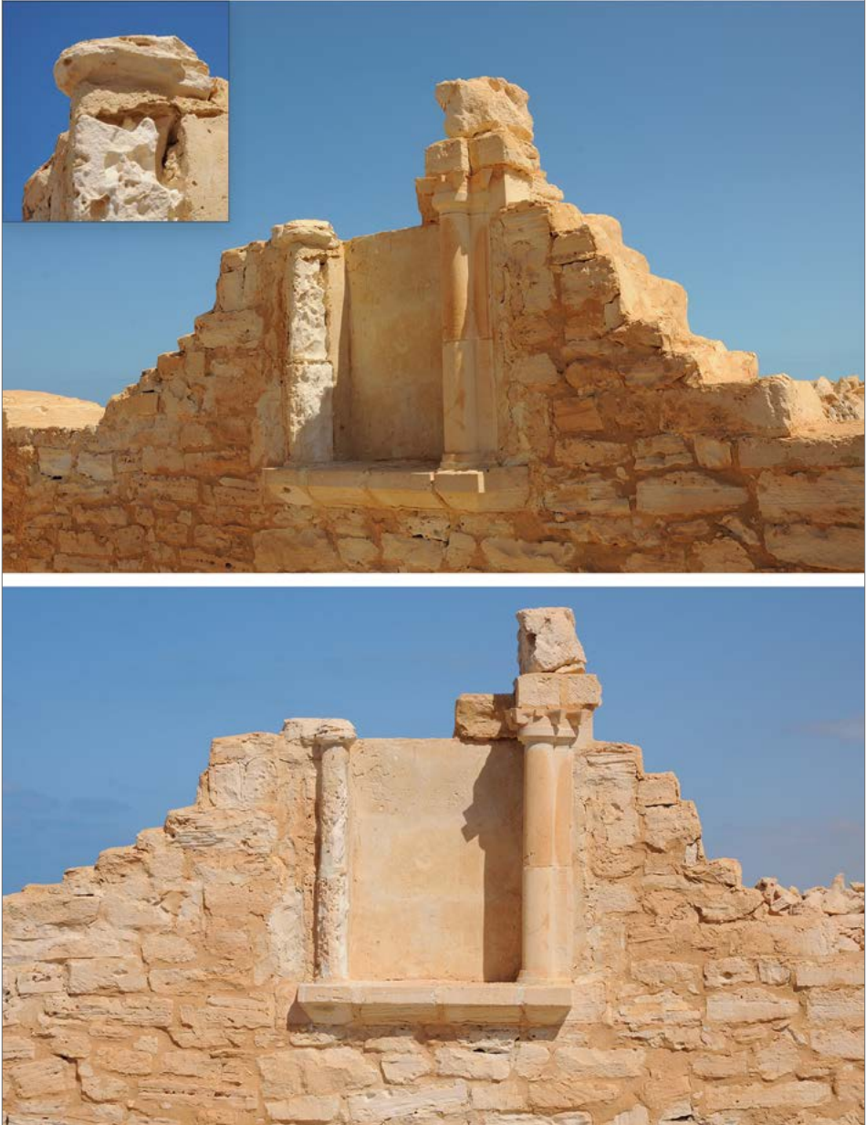
Fig. 1. Small aedicule in House H9: top, before conservation; inset, detail before conservation; bottom, after conservation (Polish–Egyptian Conservation Mission Marina el-Alamein/photos P. Zambrzycki)
