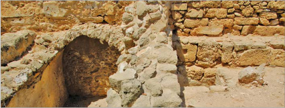
Fig. 3. Wall between rooms 13–15 on the left and 7 on the right, with plaster remains visible to the left and above the cistern (unit 15) and above a support wall in Room 7 (Photo E. Jastrzębowska, 2017)
