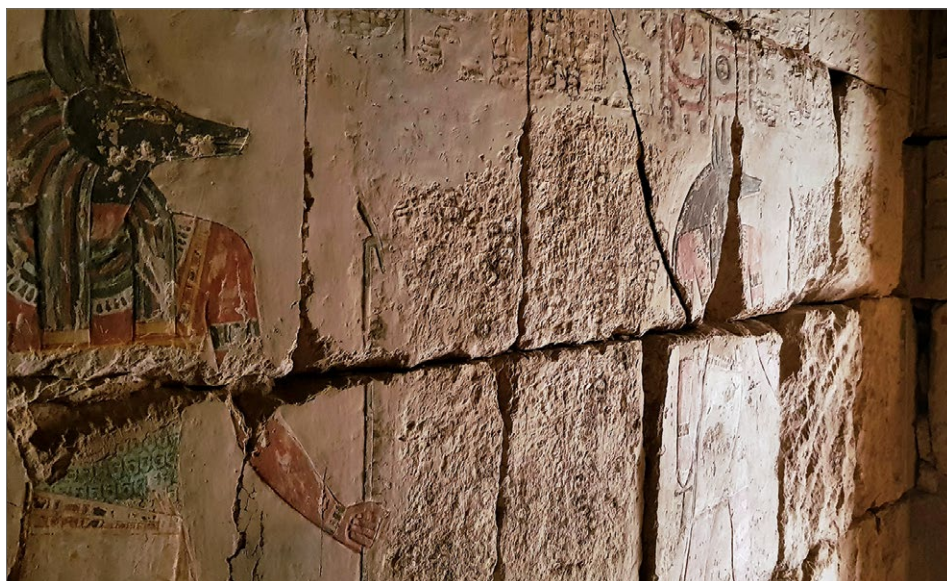
Fig. 4. The eastern wall of the Sanctuary. The wall blocks lack sharp edges, with large gaps at their joints (Photo A. Kwaśnica)
